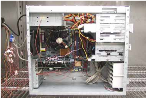
The view of the thermocouples connections.
